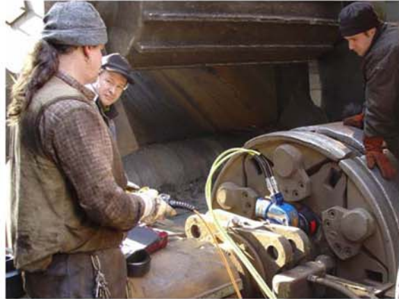
MXT-10 being used on a scrap press
